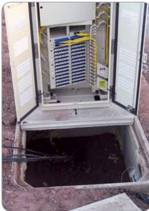
Shown with the handhole mounting option for storing slack cable, this OmniReach FDH was shipped with a 216-position fiber distribution panel and a 1x32 splitter module with splitter outputs routed to the parking lot within the cabinet.
